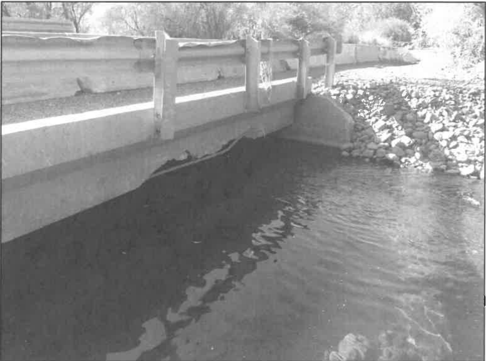
Photo 4. Damage to Bar 14 Road Bridge.
