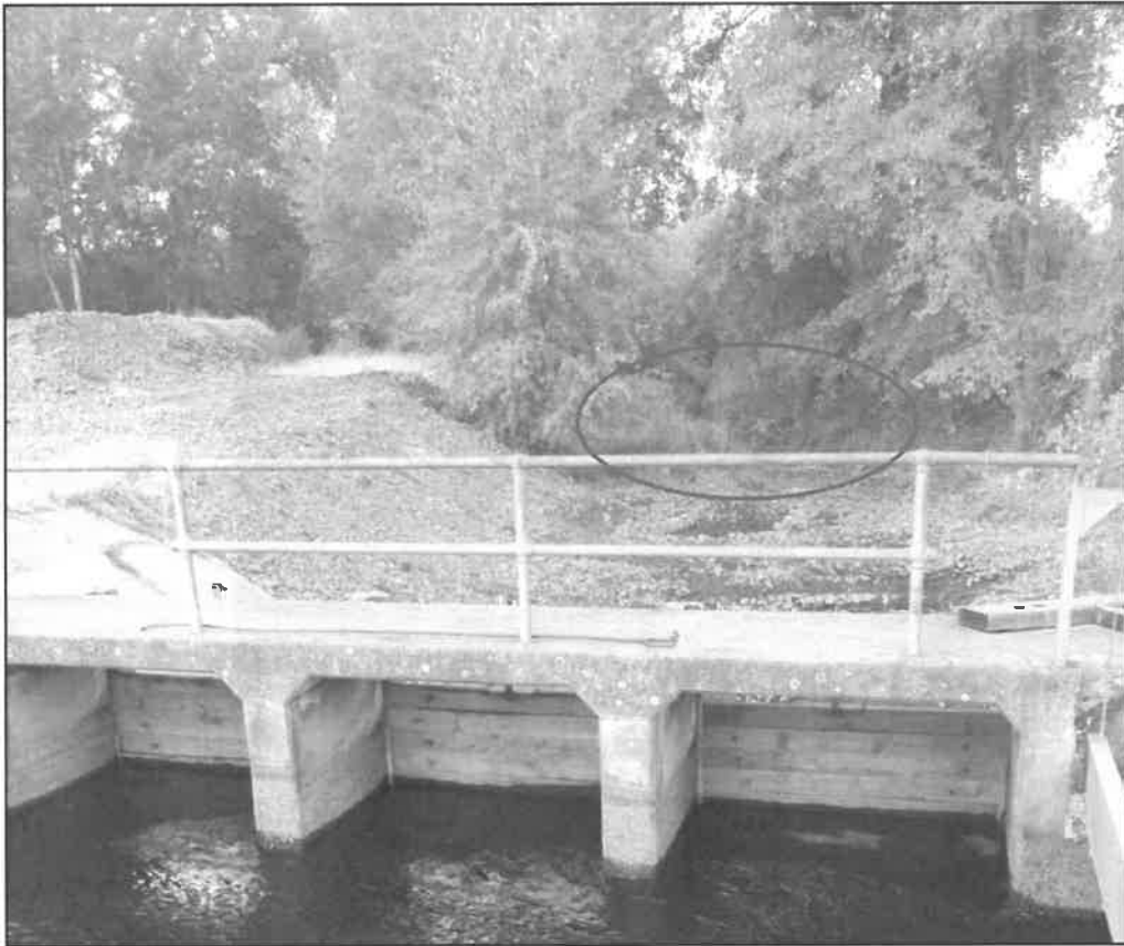
Photo 1. KRD intake looking upstream at Naneum Creek channel. Note chronic bedload on the left that is removed from the intake structure. Circle shows perched bedload.
